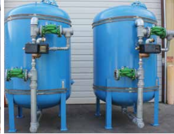
Twin 60"x60" Progressive Flow Water Softeners with 4" service valves and Fleck 3150 regeneration valves.
